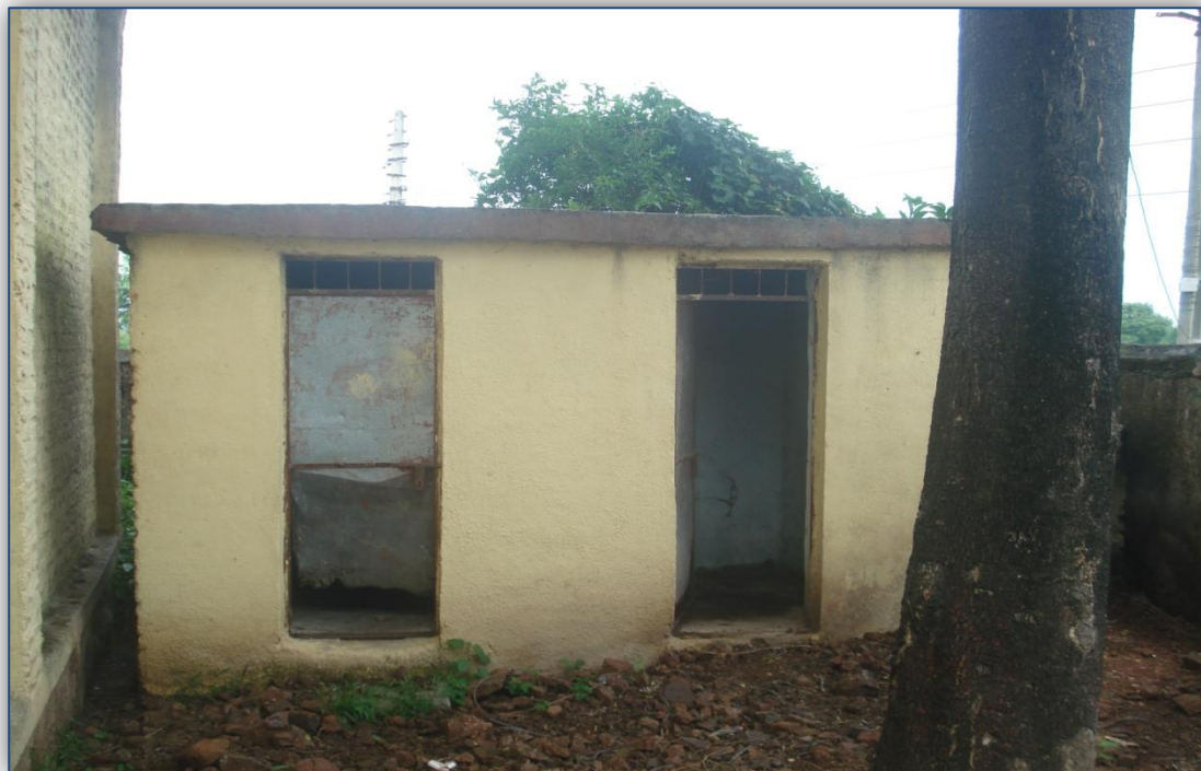
Toilet: Not cleaned and maintained properly.
